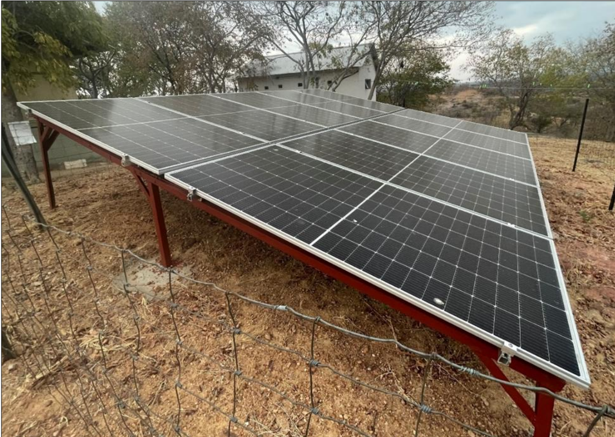
Figure 18-84: GoviEx Muntanga camp ground-mounted solar panels
