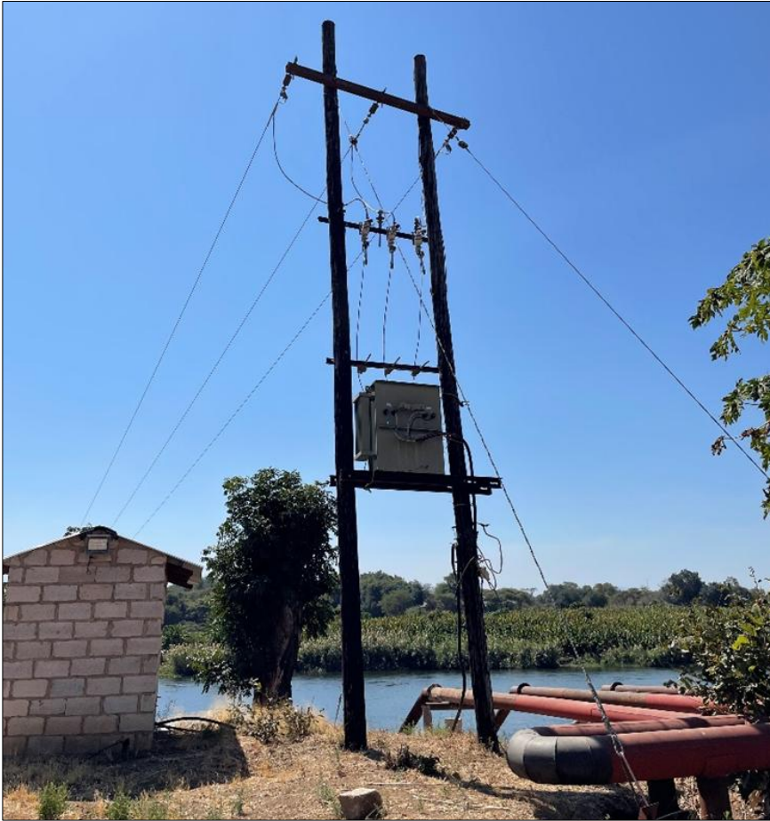
Figure 18-83: 11 kV line terminus at Palabana fish farm
