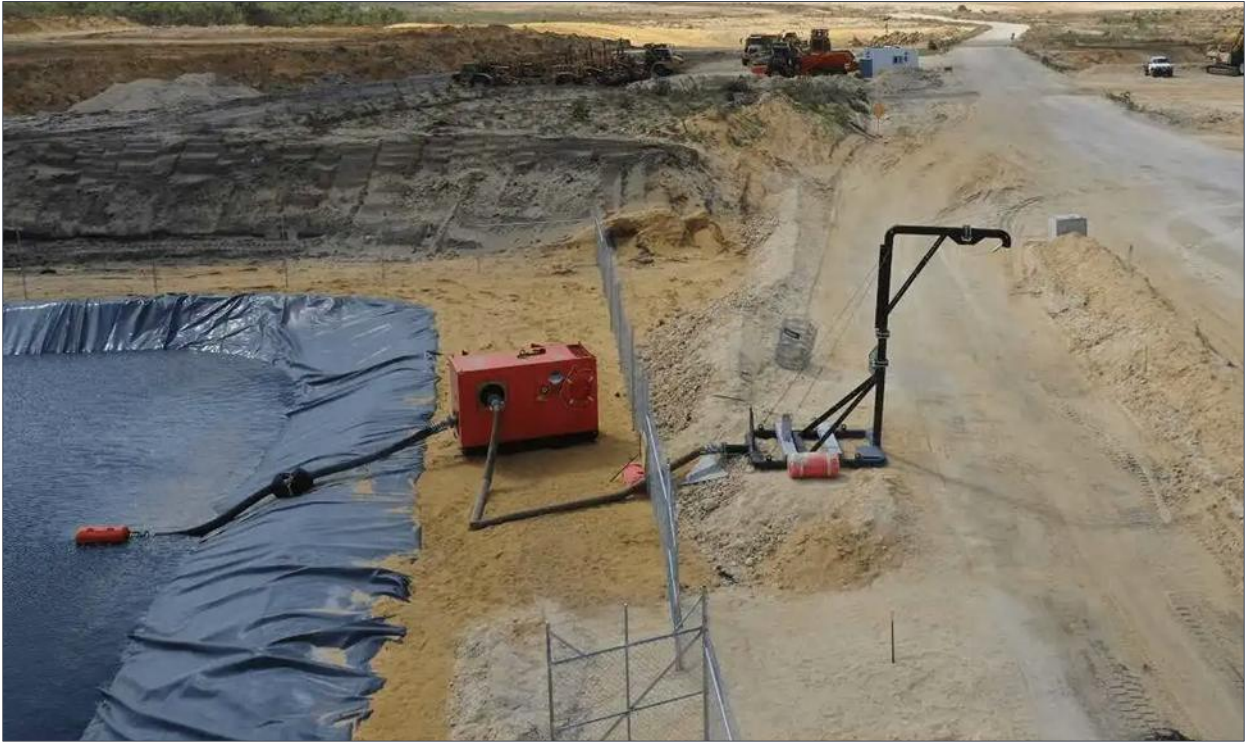
Figure 18-39: Typical dust suppression filling standpipe
